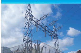
Biomass power plant
